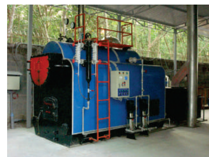
STEAM BOILER FOR DRYER AND STEAMER
